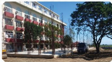
Construction of College of Public Administration and Governance Building Lucinda Extension Campus (Phase I)
