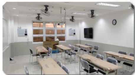
Refurbishment of Classrooms and Laboratory Rooms (Phase III) College of Public Administration and Governance
